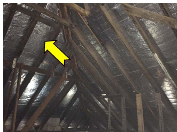
Photo 6. Interior, roof space, throughout – suspected SMF sarking insulation.
