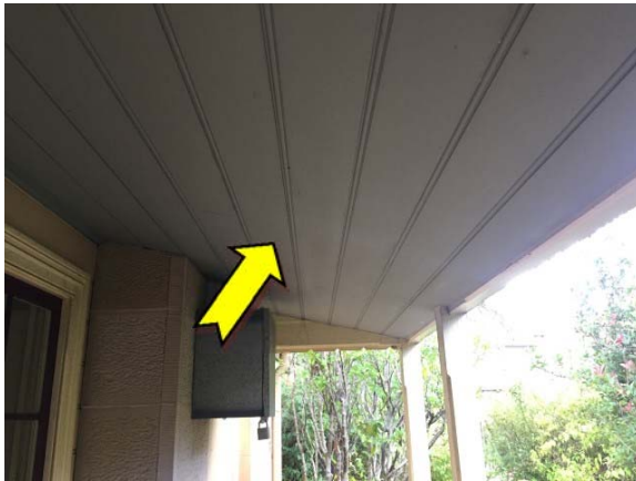
Photo 9. Exterior, throughout, awning – suspected lead-containing light green upper paint system.
