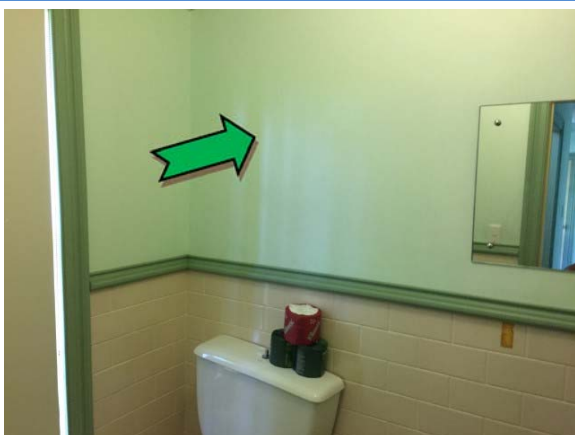
Photo 5. Interior, toilets, walls – non asbestos-containing fibre cement sheeting and grey mastic sealant.
