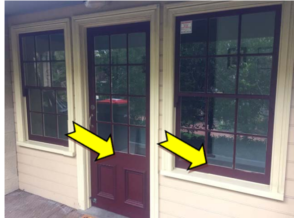
Photo 8. Exterior, throughout, window and door frames – suspected lead-containing red upper paint system.
