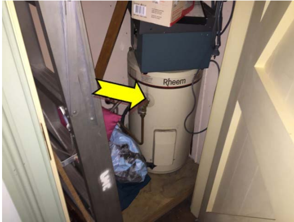
Photo 7. Interior, south elevation, east cupboard, hot water heater – suspected SMF internal insulation.
