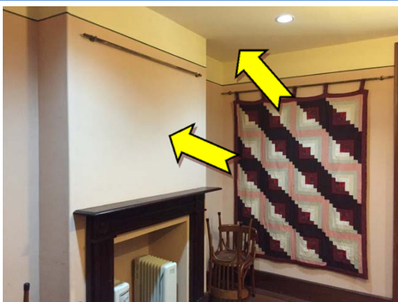
Photo 11. Interior, rooms 1 and 2, walls, upper level walls and ceiling – suspected lead-containing pink and cream upper coloured paint systems.
