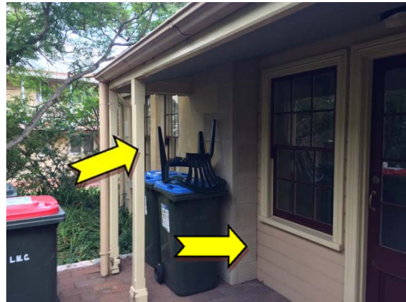
Photo 10. Exterior, throughout, walls, columns and features – suspected lead-containing yellow and beige upper coloured paint systems.
