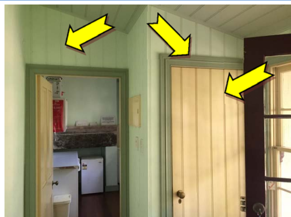
Photo 12. Interior, hall and back of house, walls, ceiling door and frames – suspected lead-containing light green, dark green and yellow upper coloured paint systems.
